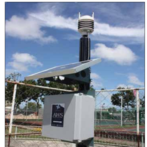
Additional rain gauges were installed in CAMANAVA recently.
