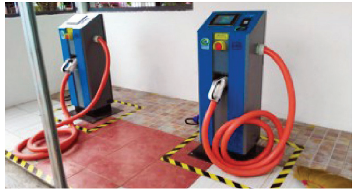
CharM charging station in Cauayan City, Isabela
